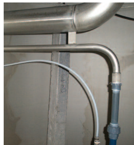
Fig. 2. The rod-shaped magnesium anode is clearly visible in the filter unit of a stainless steel ozone reaction tank (photo by Innomet B.V.).
