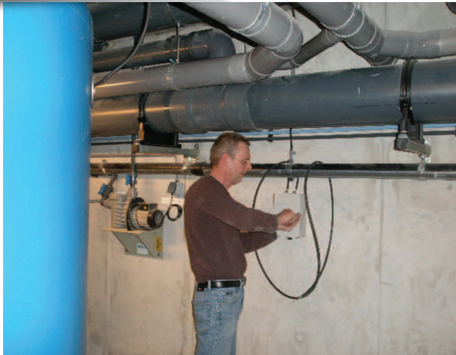
Fig. 1. Installation of an intelligent cathodic protection system in a stainless sand bed filter (photo by Innomet B.V.).
