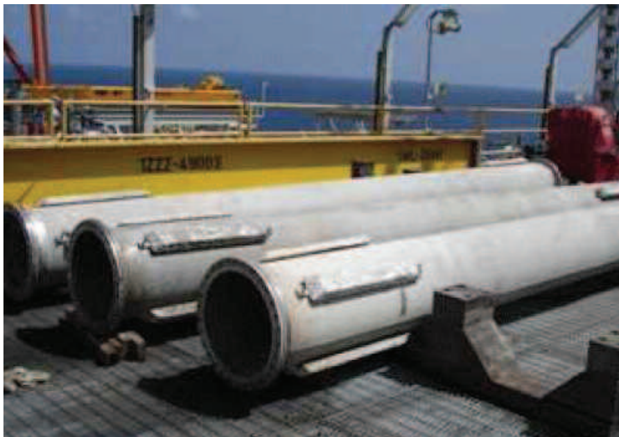
Fig. 6. Over protected duplex stainless steel (1.4462) risers protected by conventional cathodic protection with cracks in the weld
