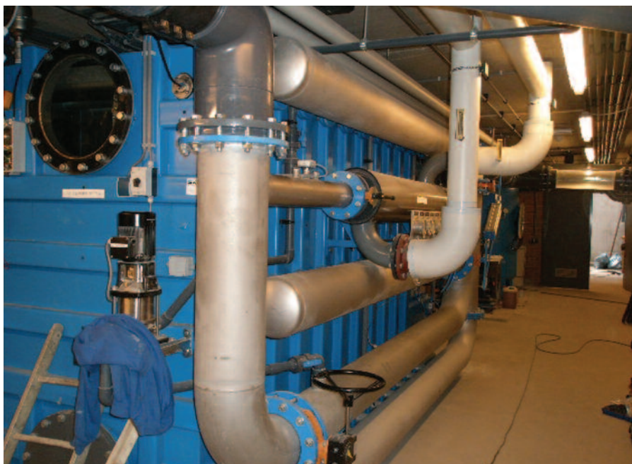
Fig. 3. Stainless steel sand bed filters used for cleaning swimming pool water are also protected using intelligent cathodic protection (photo by Innomet B.V.).
